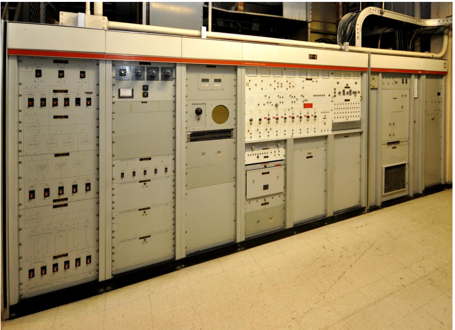
Collins Radio 821A-1, 250 KW, Transmitter
